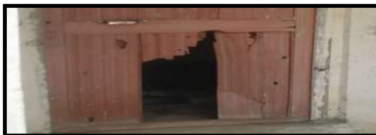
Fig 8: Poor Toilet Condition In Public School
