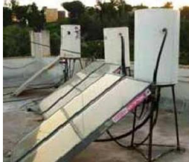
Fig.1. Solar water Heater
