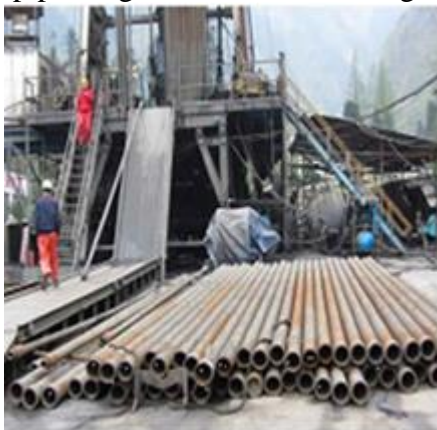
Figure 1: The worker pushes a string along the catwalk using pneumatic winch steel rope.
