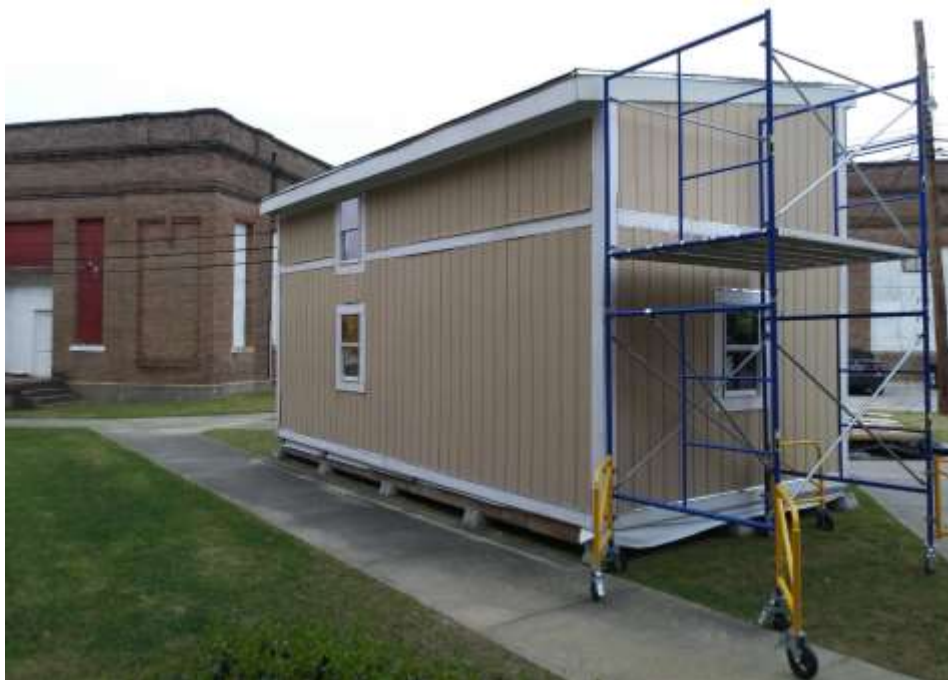
Figure 2: Tiny house with finished walls and windows. A movable scaffold is still in place for wall painting operation. See the worker platform for higher or elevated reach during wall painting.
