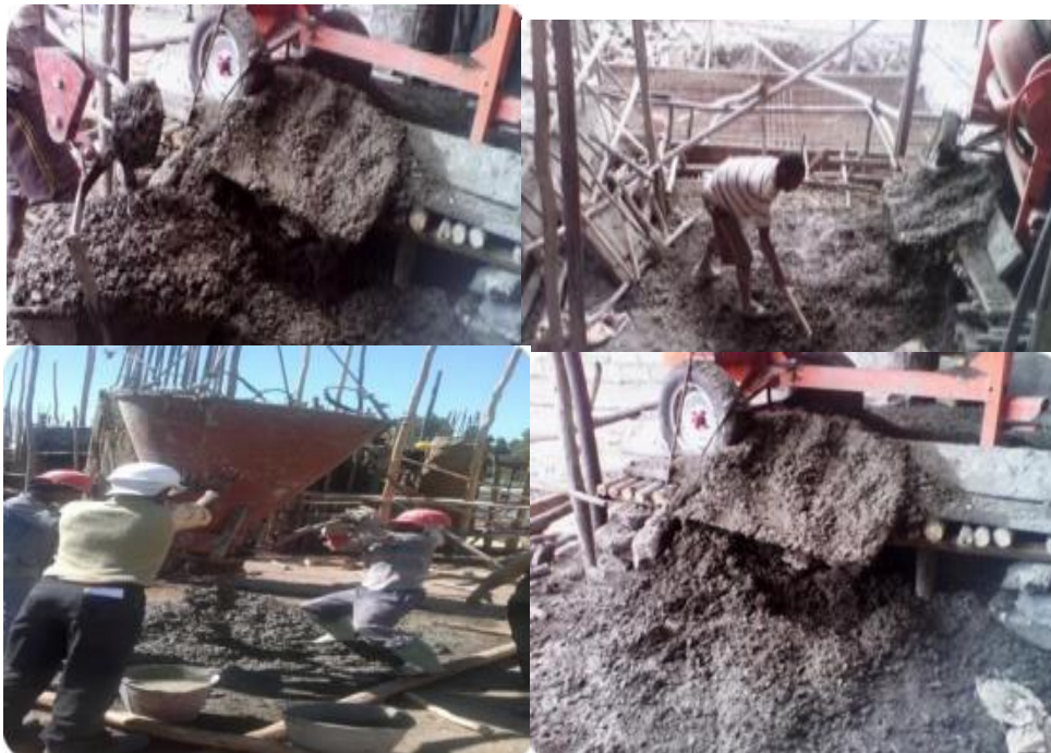
Figure 4.6: Wastage of concrete due to Poor transport on site at Aflao Source: Field research
