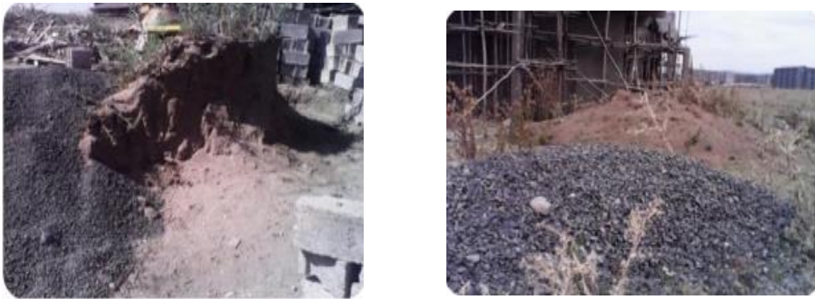
Figure: 4.5 Poor handling of Coarse aggregate on construction site at Jasikan Source: Field research
